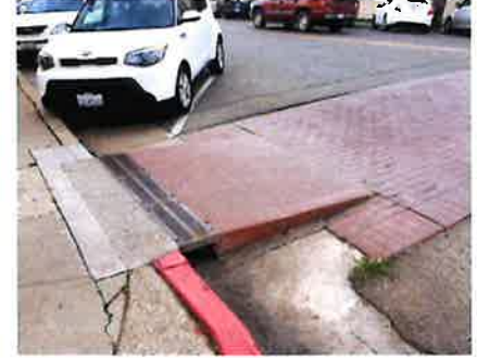
PEDESTRIAN CROSSWALKS WITH CONTRASTING PAVEMENT
